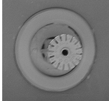
Wet sprinkler head
